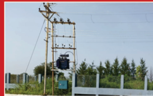
Transformer & Street Light
